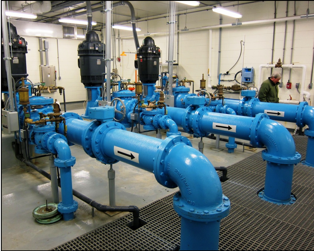
High-lift pumps inside the Glenville Water Treatment Plant
