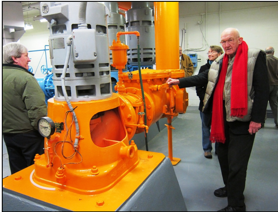
Committee members tour the inside of the Water Treatment Plant
