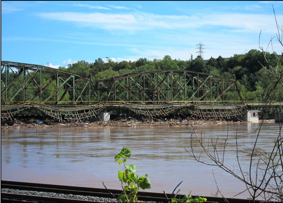
Damage and debris at Lock 10 following Tropical Storm Irene in August, 2011
